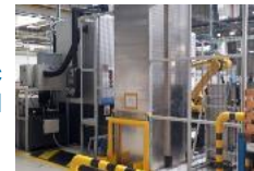
Automatic Turning Cell
